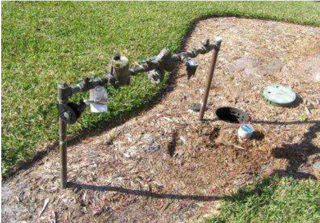
Secondary irrigation system at cul-de-sacs. Controller located in hand hole.
