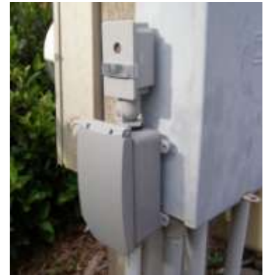
Entry island photocell and duplex outlet on side of distribution panel
