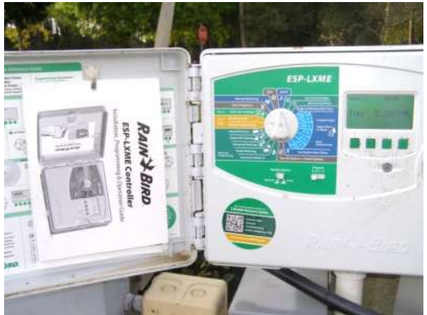
Primary irrigation control panel
