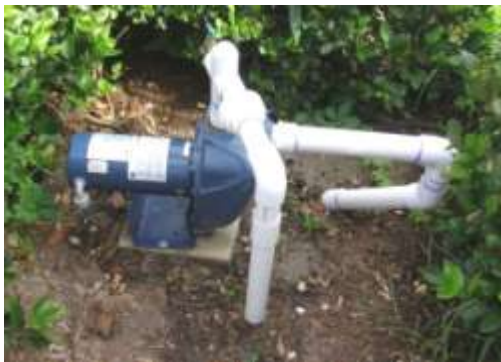
Irrigation pump and motor
