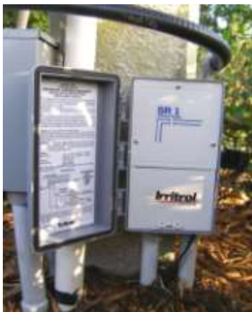
Irrigation pump starter
